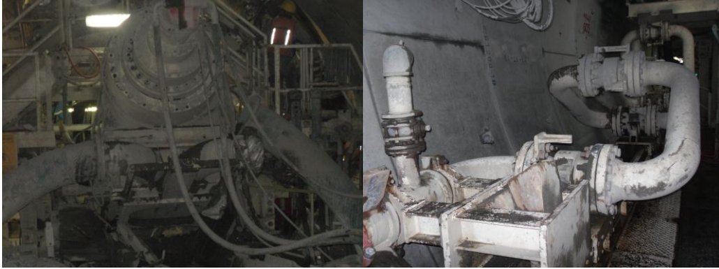
Figure 3. Schwing pumps TAP-140 used in the Herrenknecht TBM
